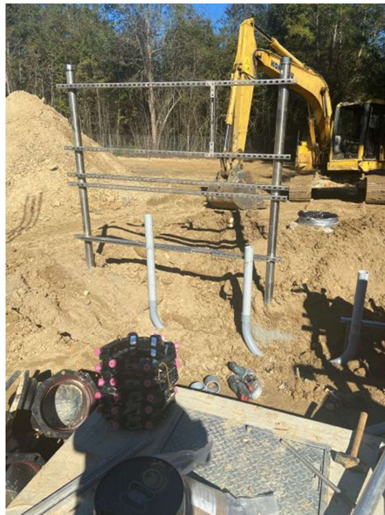
Photo 1: Control panel pad
